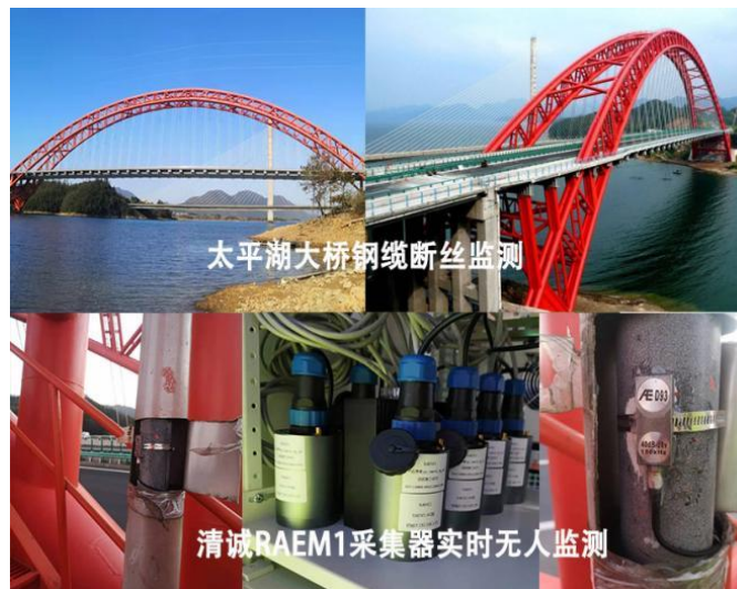
Taiping Lake Bridge steel cable broken monitoring site
